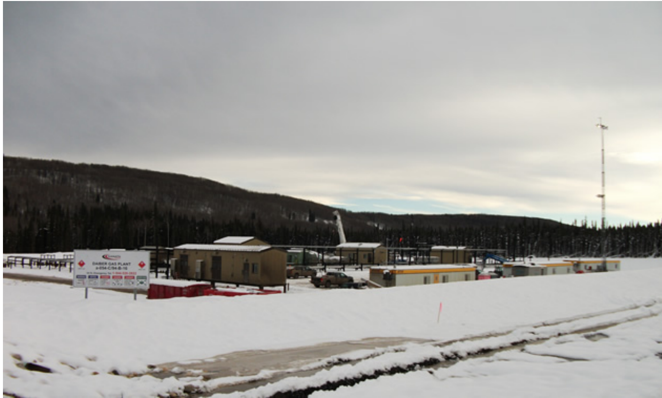
KANATA Energy Group's site north of Fort St. John is now under construction. — Photo courtesy KANATA Energy Group
